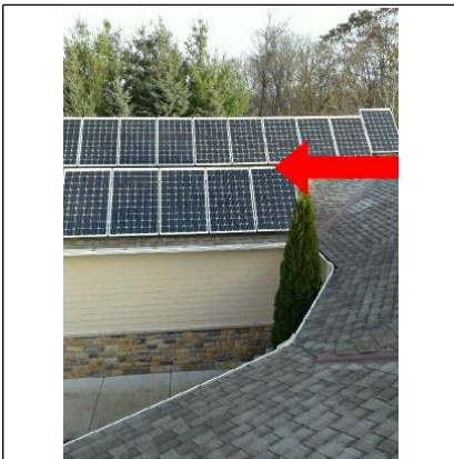
Bank of solar panels.
