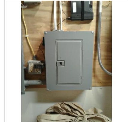
This box was put in for a generator. The generator has never been installed.
