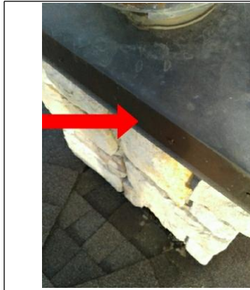
There are a few loose Nails around the chimney cap. They should be pound it in.
